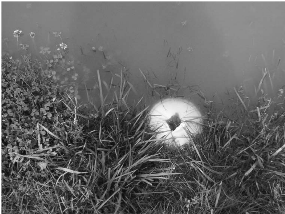
Water from a nearby retention pond is seeping into this broken cleanout cap. The WCCD asks Avon residents to look for problems like this and report them to the WCCD. This broken cap is causing water flow that takes up space needed to carry sewage to the treatment plant.
